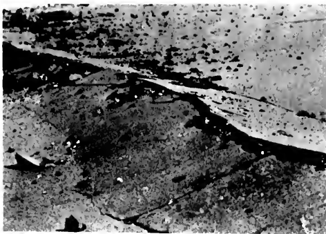
Photo 25. Buckled asphalt pavement caused by large compressive ground deformations.
